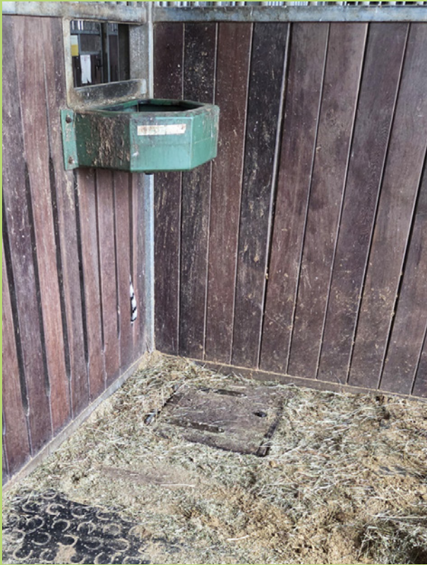
Chain-driven manure removal system at the Tennenlohe riding stable
